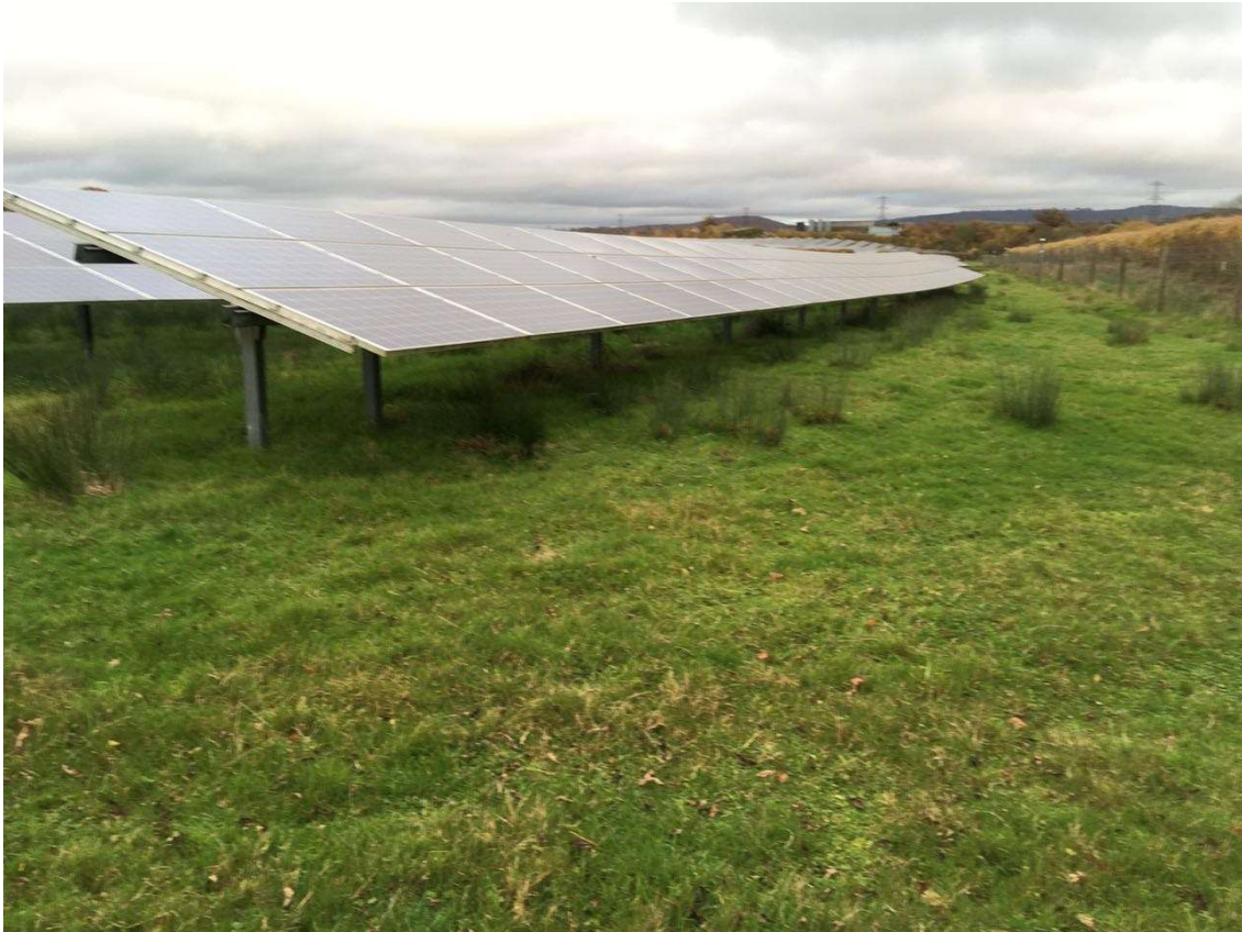
Figure 6-16-1 Drainage of solar panels onto grass
