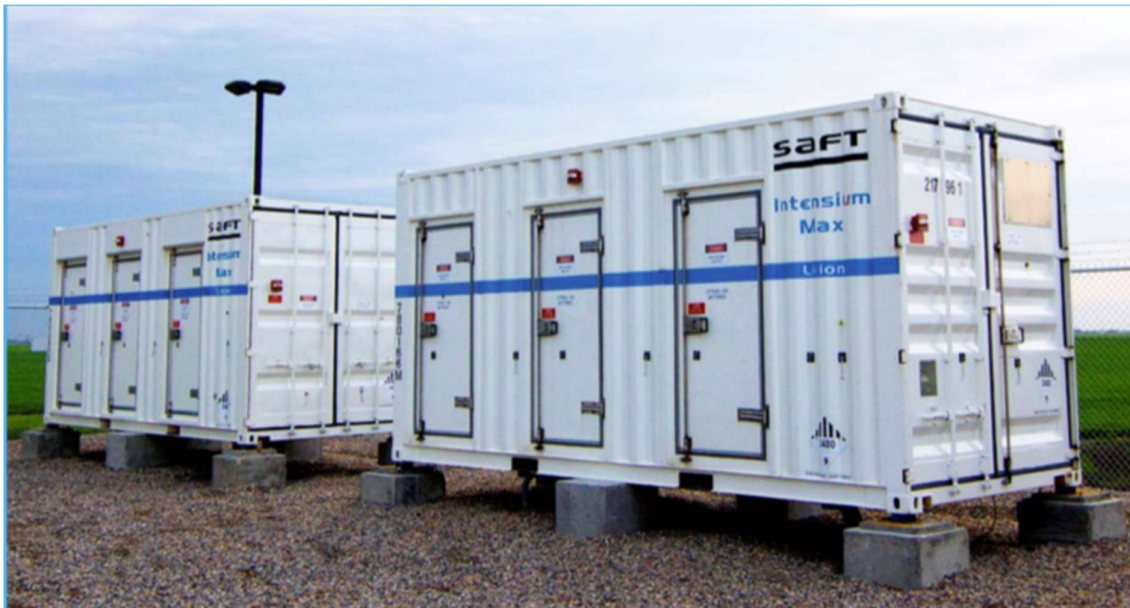
Figure 6-26-2 Typical battery containers used on a solar farm
